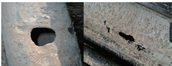
Figure 3 Casing Corrosion Punching
