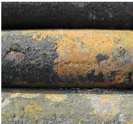
Figure 1 External Corrosion of Casing
