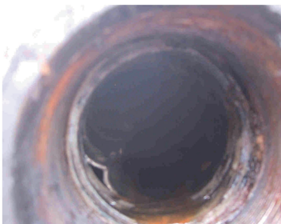
Figure 2 Internal Corrosion of Casing
